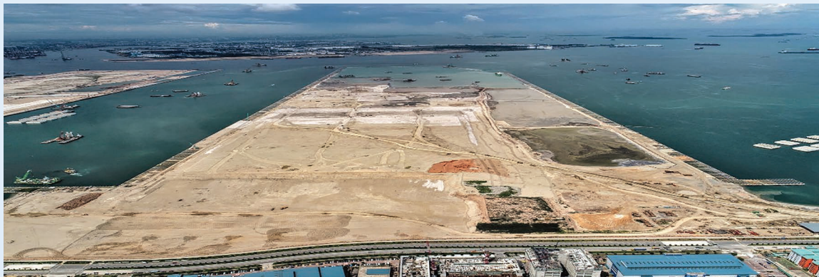
▲ Sustainability is integral to the construction of Tuas Port. More than 50% of the fill materials for Tuas Port Phase 1 reclamation were either dredged from the creation of port's fairways or excavated from other construction projects on land.
